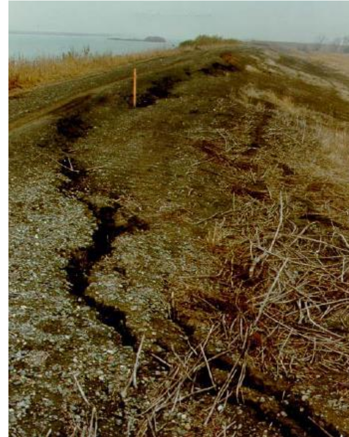
Levee crown cracking due to slope instability during flood event
