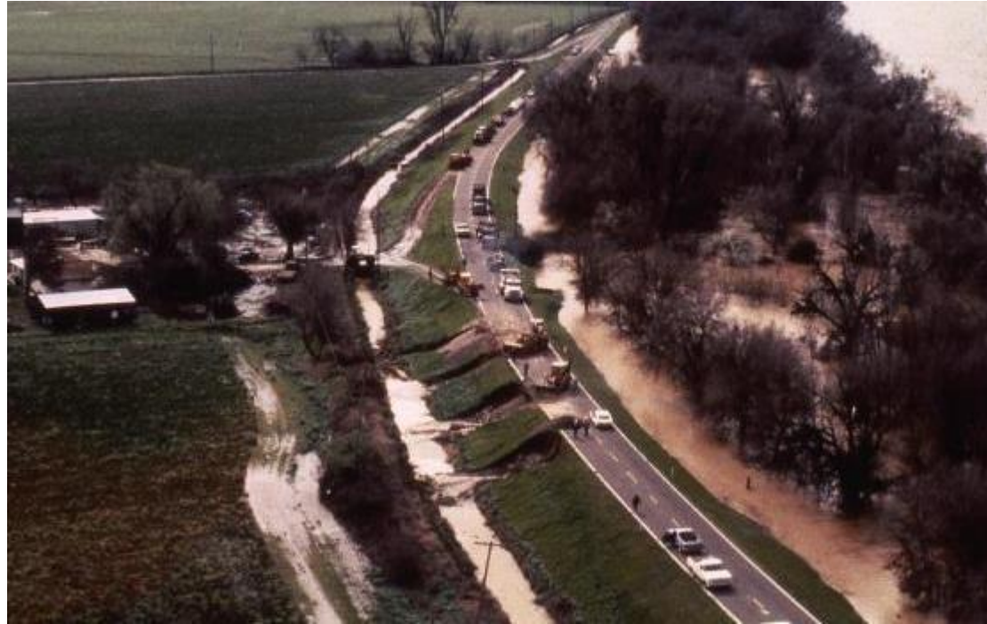
Landside levee distress during flood event - sloughing caused by through-levee seepage.
